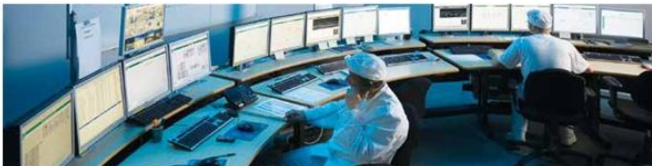
Process control room
