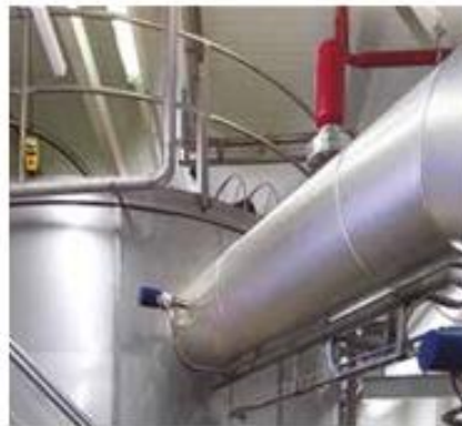
GEA Spray dryer - side view
